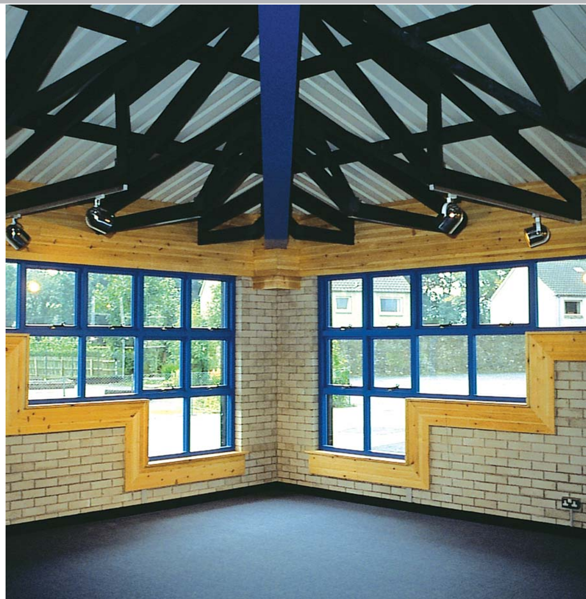
Roof trusses finished with tinted Kiva Interior semi-matt Lacquer. Redwood lining boards to wall areas finished with Kiva Interior semi-gloss Lacquer.
